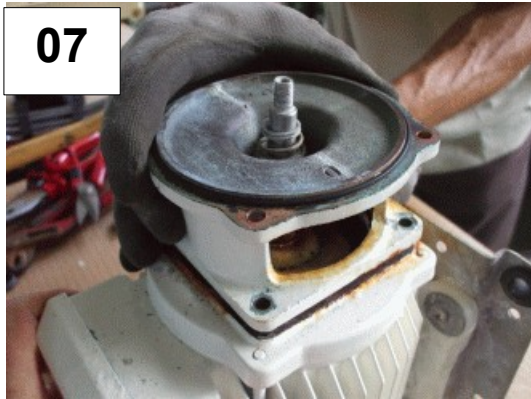
07 Removal of the back pump body together with the old shaft seal
